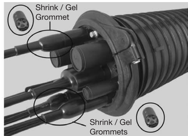
Accommodation of fibre optic cables in connection with a Corning mechanical closure
